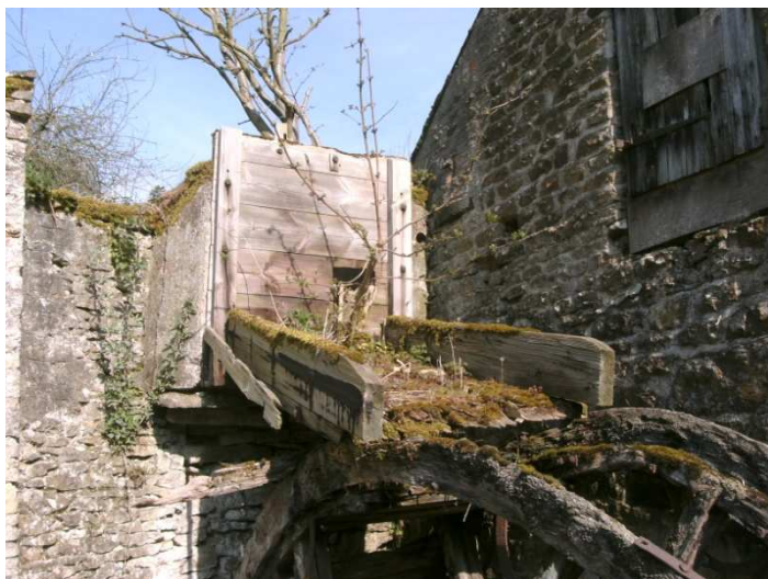
trough and plank penstock
