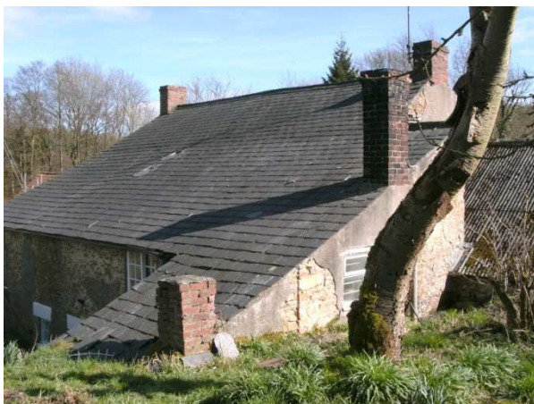
back, cat-slide roof of the house, some remnants of opc render
