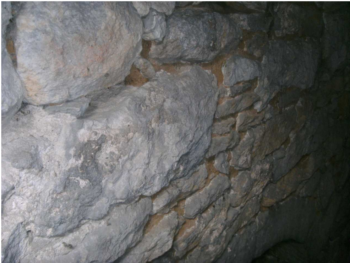
Earth mortar within tower(above) and same, with original lime pointing, Pond Farmhouse
