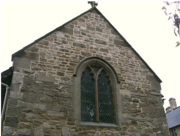
Repointing of gable and of areas of loose opc at lower level.
